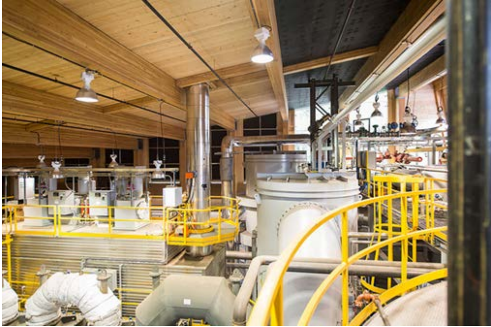
Figure 2 Interior view of the BRDF.
