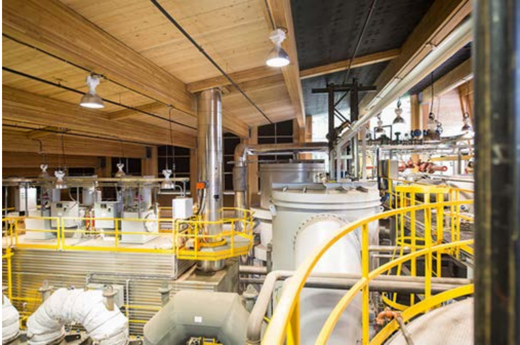
Figure 2 Interior view of the BRDF.
